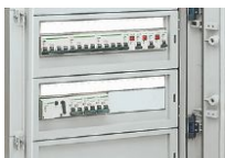
Detail from the circuitmarking system.
